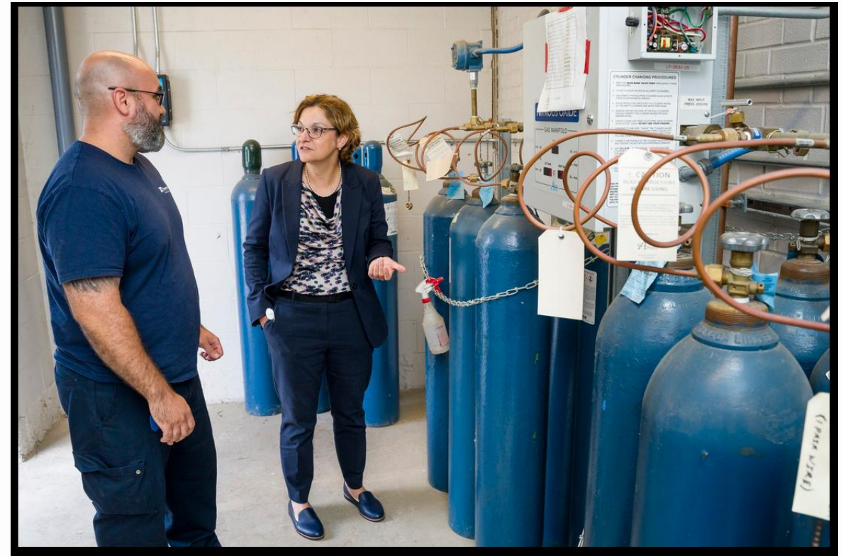
Back-up system in the tank room Holland Orthopedic Centre – Tanks only
