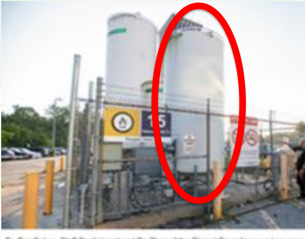
5000 Kg external bulk tank – temperature and pressure sensitive
